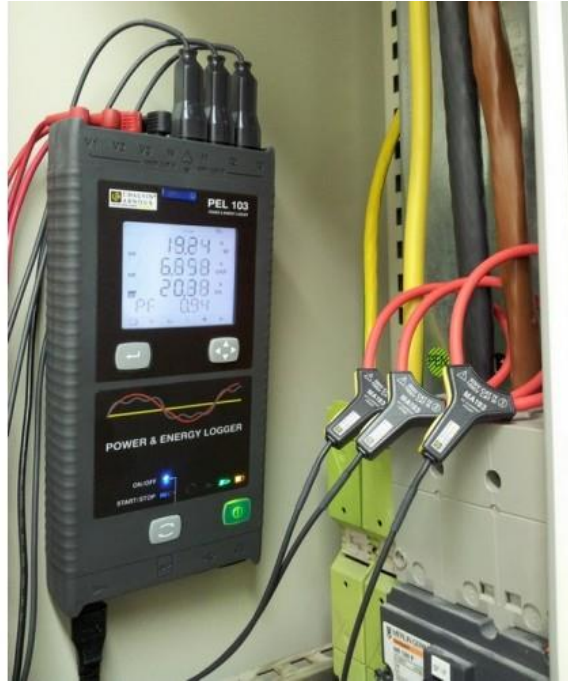
Figure 10: Measurement method of energy consumption, power factor, and power harmonics tests.
